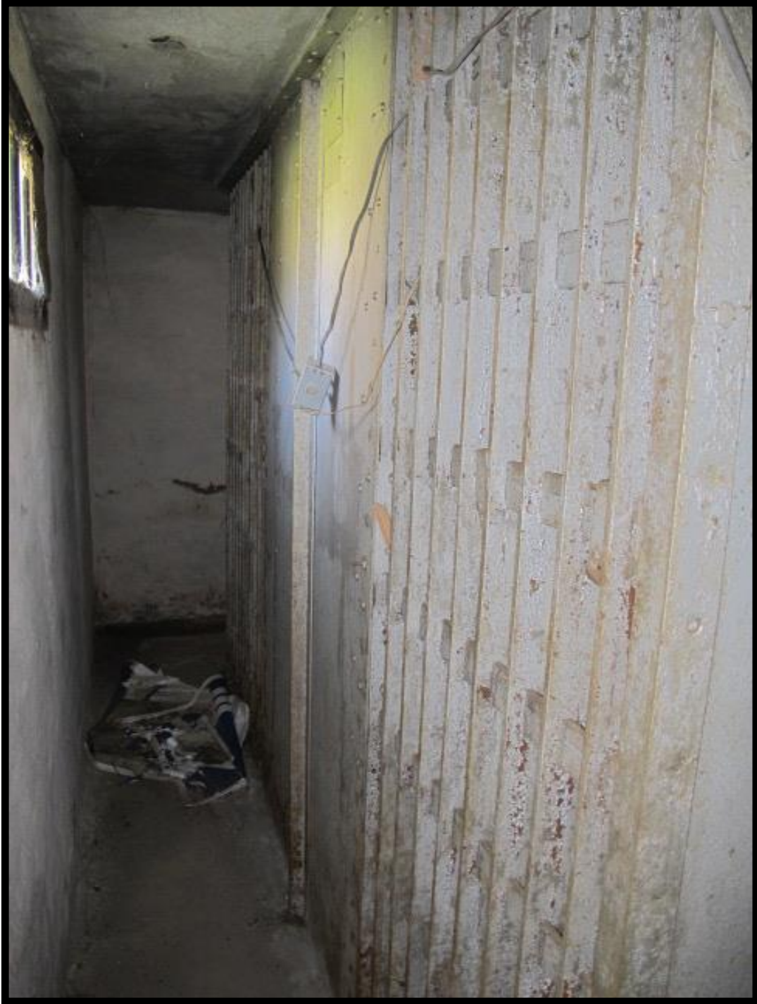
Figure 2.2-41: Huntersville Town Jail (MK3299), View of Rear Wall of Cell Block Looking East.
