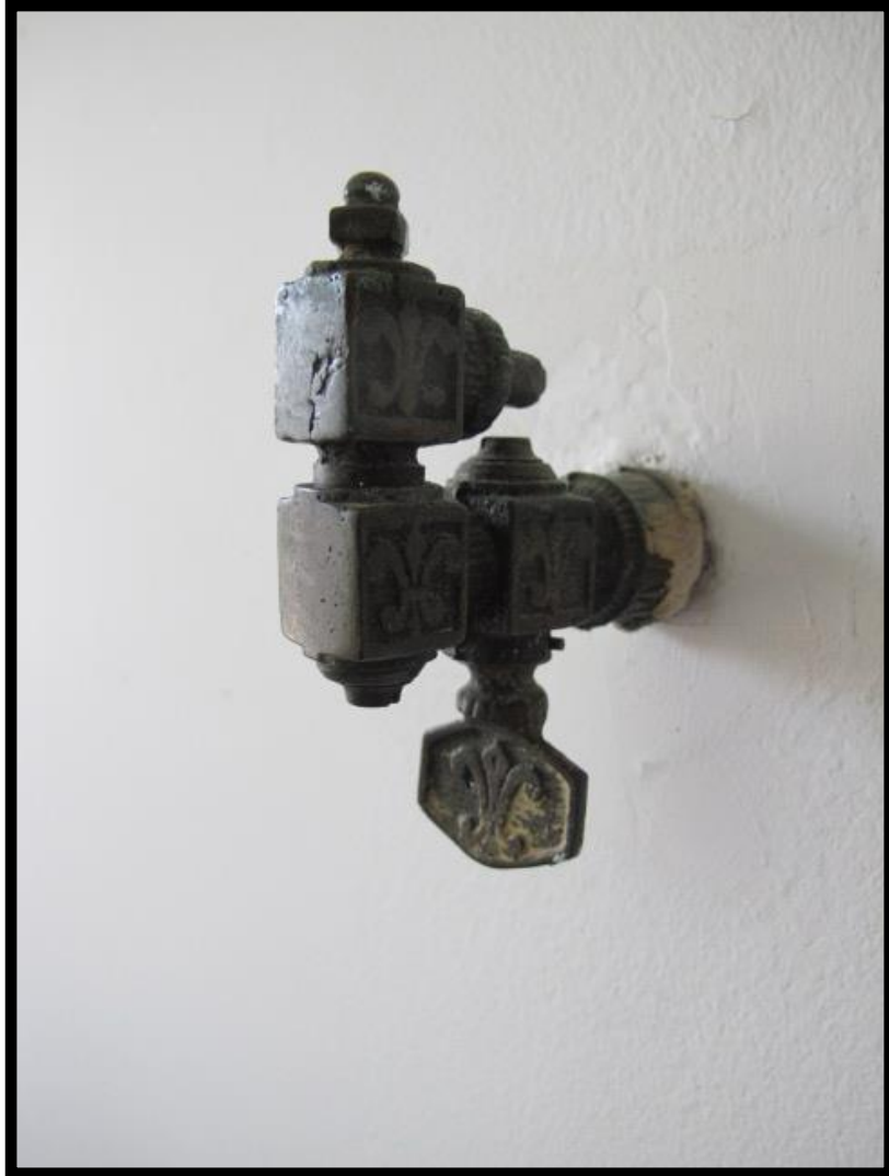
Figure 2.2-23: Ranson House (MK1351), Only Surviving Original Gas Fixture in Second Floor Bathroom.
