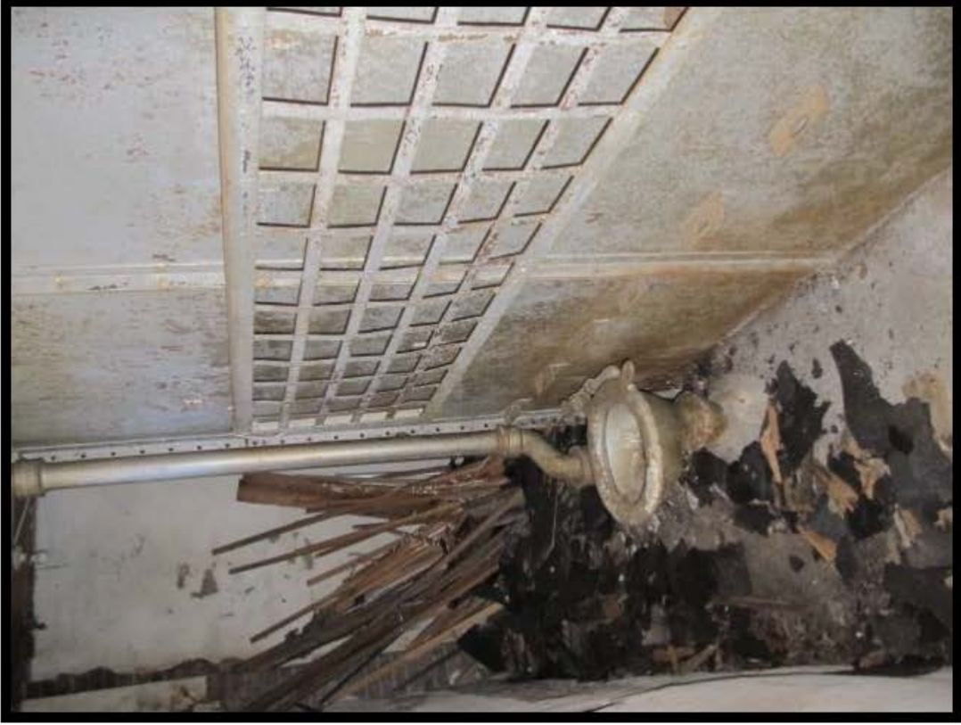
Figure 2.2-40: Huntsville Town Jail (MK3299), View of Ancillary Bunk and Toilet Looking South.
